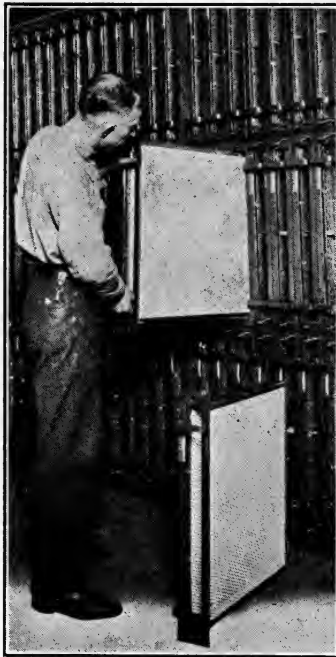
FIG. 7. Airmat filters installed in West Coast studio.
